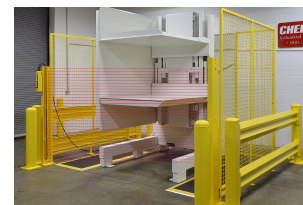
SAFETY DEVICES: Light curtains, safety mats and laser scanners protect the front of the machine for additional protection
